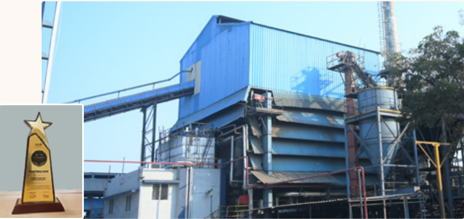
Biomass boiler at Digwal, India
