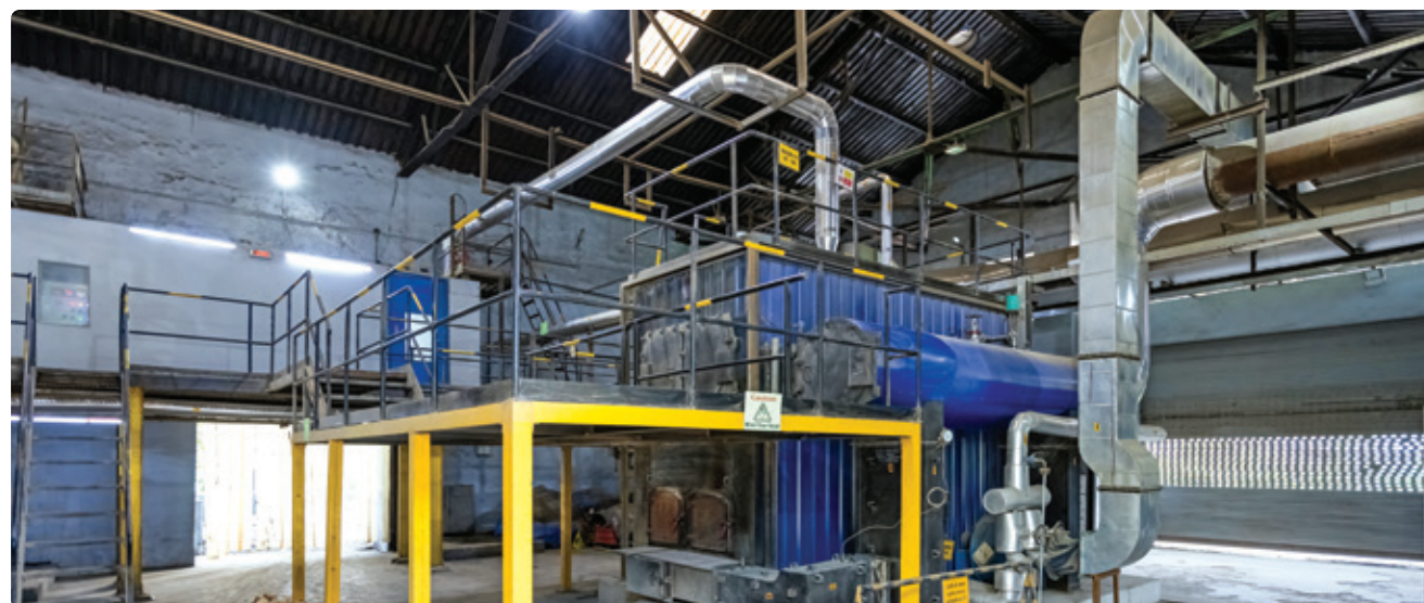
Biomass boiler, Pithampur, India
